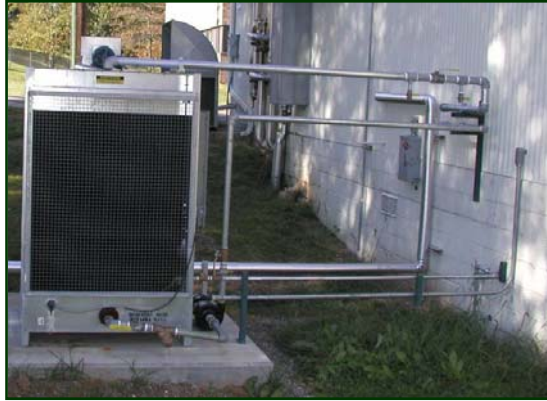
Cooling Tower for 10-Ton (35-kW) Single-Effect Absorption Chiller
